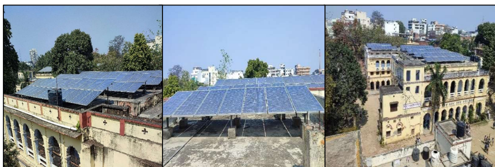
Figure 5: Rooftop Solar Panels
