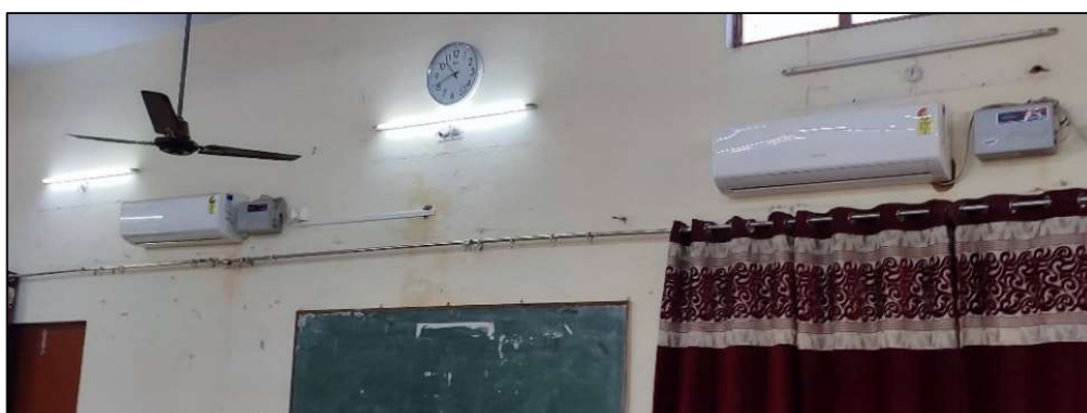
Figure 6: Energy saving 3-star AC installed in the Hall
