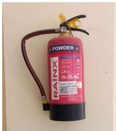
Figure 8: ABC-MAP 90 type Fire Extinguisher installed at each floor of the campus building
