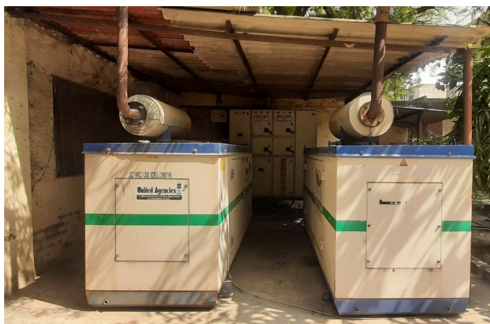
Figure 4: DG sets for Electricity Backup
